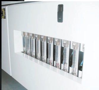
Gas Flow controls thanks to flowmeters.
